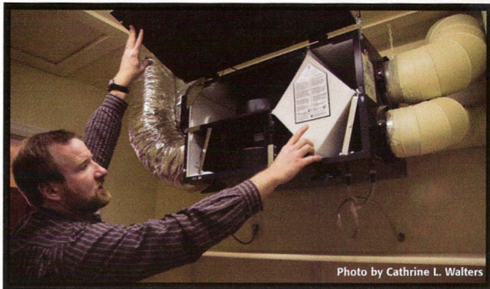
The I-Pad's Heat Recovery Ventilator maintains a consistent climate and moisture content inside the house.
